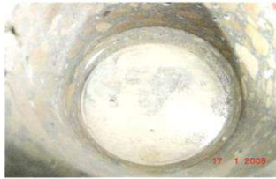
Photo No. 6: A Close View of the Core Hole in the Floor Slab.
