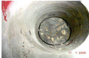
Photo No. 4: A Close View of the Core Hole in the Column.
