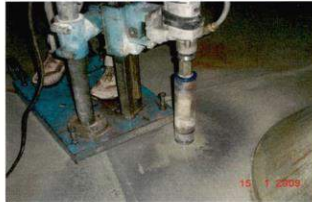
Photo No. 2: A Close View of Extraction of Core from Column Footing.
