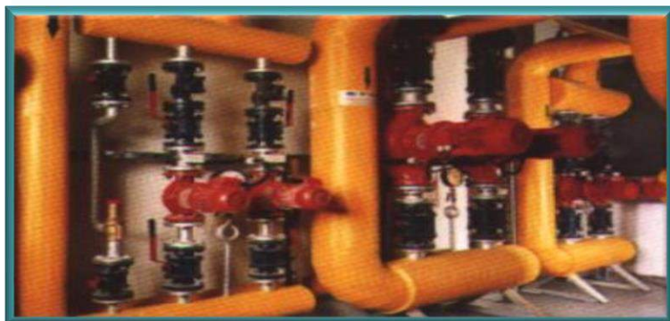
Sub - Station, Jeddah - KSA
