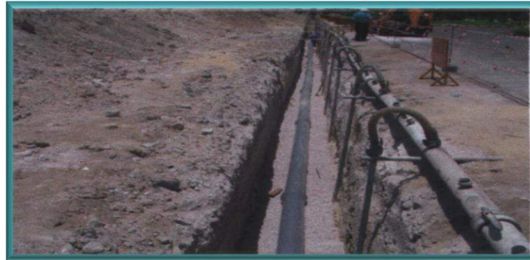
Waste Water Piping, Dammam - KSA
