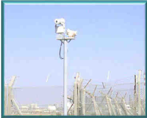
Security System PTZ Camera for Yanbu Commercial Port, Yanbu - KSA
