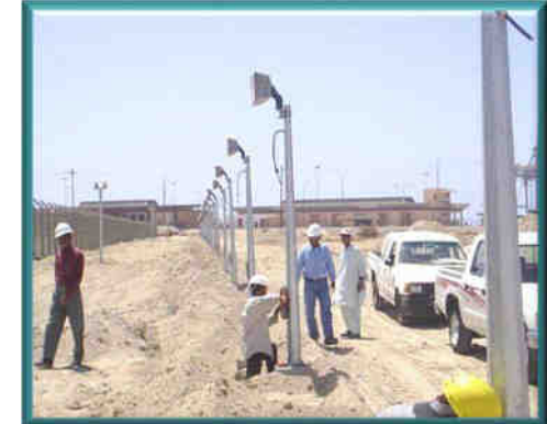
Security Lighting System for Yanbu Commercial Port, Yanbu - KSA
