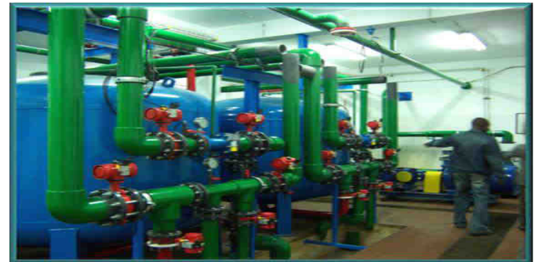
Khursaniyah Gas Plant, Jubail - KSA
