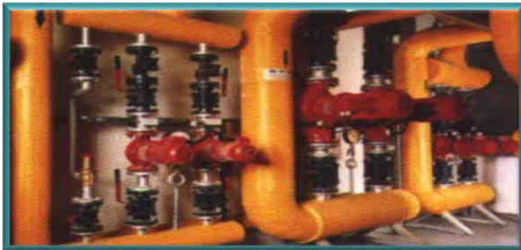
Sub - Station, Jeddah - KSA
