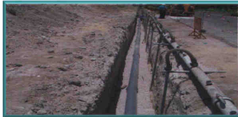
Waste Water Piping, Dammam - KSA
