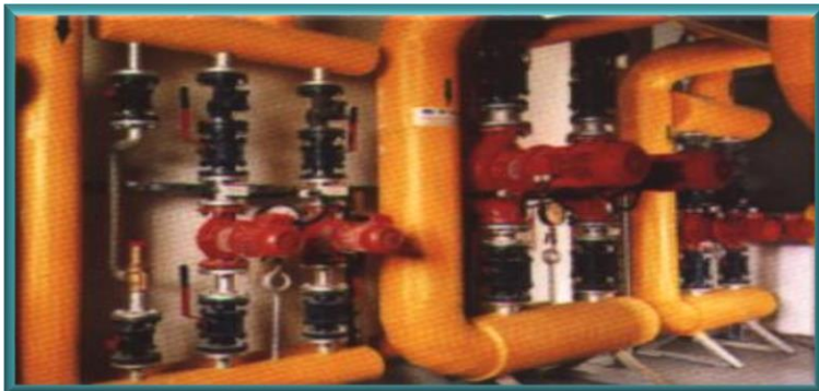
Sub - Station, Jeddah - KSA
