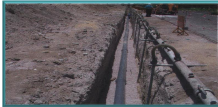
Waste Water Piping, Dammam - KSA
